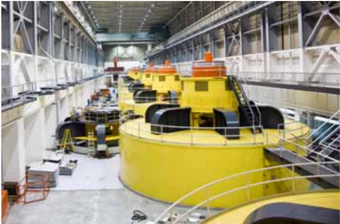
Hydroelectric power generators
